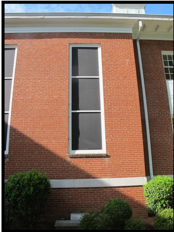
Figure 2.2-3: Detail of North Wall of Church (MK1342), Showing Window Screen and Water Table.
